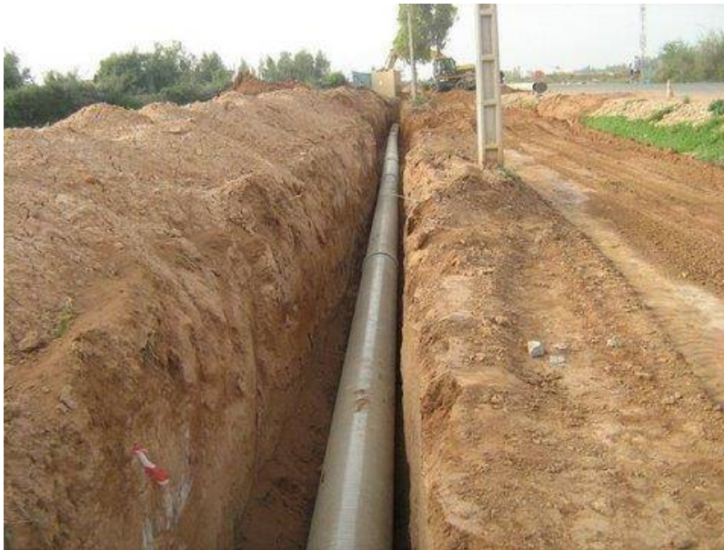
Figure 30: El Guerdane irrigation pipeline
